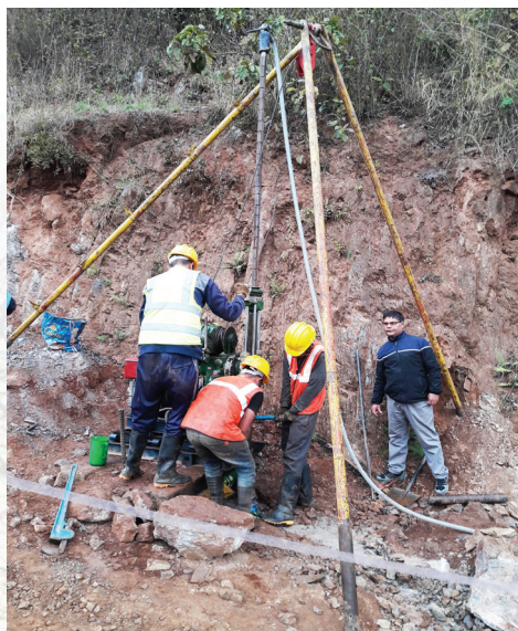
Soil testing being conducted at Benighat-5 of Dhading district, a site along the route of transmission tower construction on 27 February 2019.
