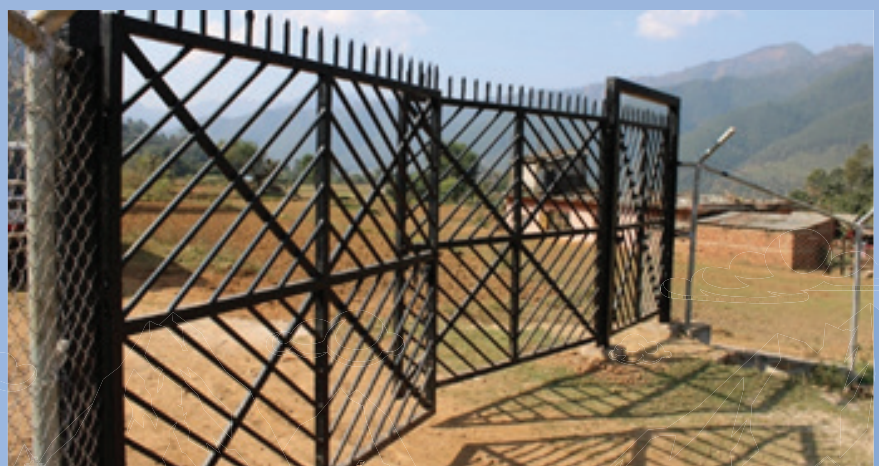
The Completed boundary wall fence around 20.27 hectares of land at the Ratmate Substation construction site in Belkotgadhi, Nuwakot.
