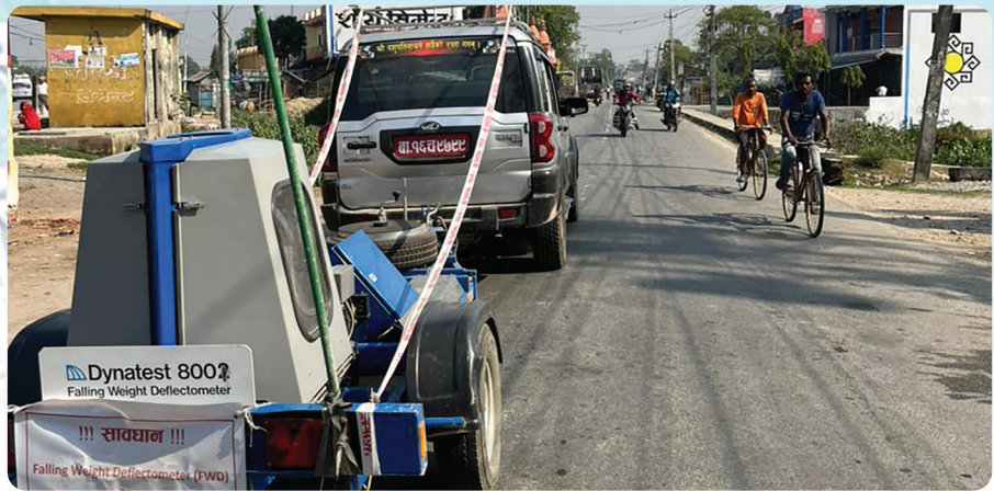
The deflection of road pavement at Kanchanpur in Saptari district being measured using FWD equipment on 29 March 2023.
