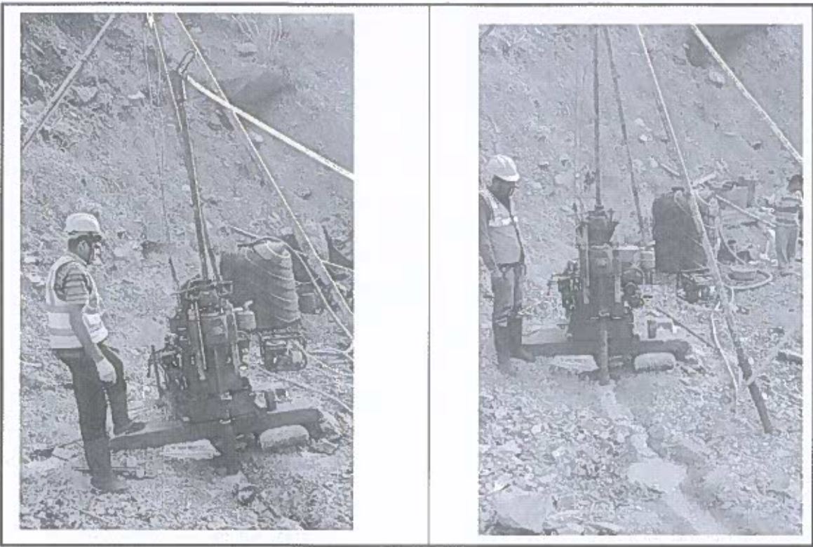
Photograph: Drilling works is progressing with the water return from the Borehole B31
