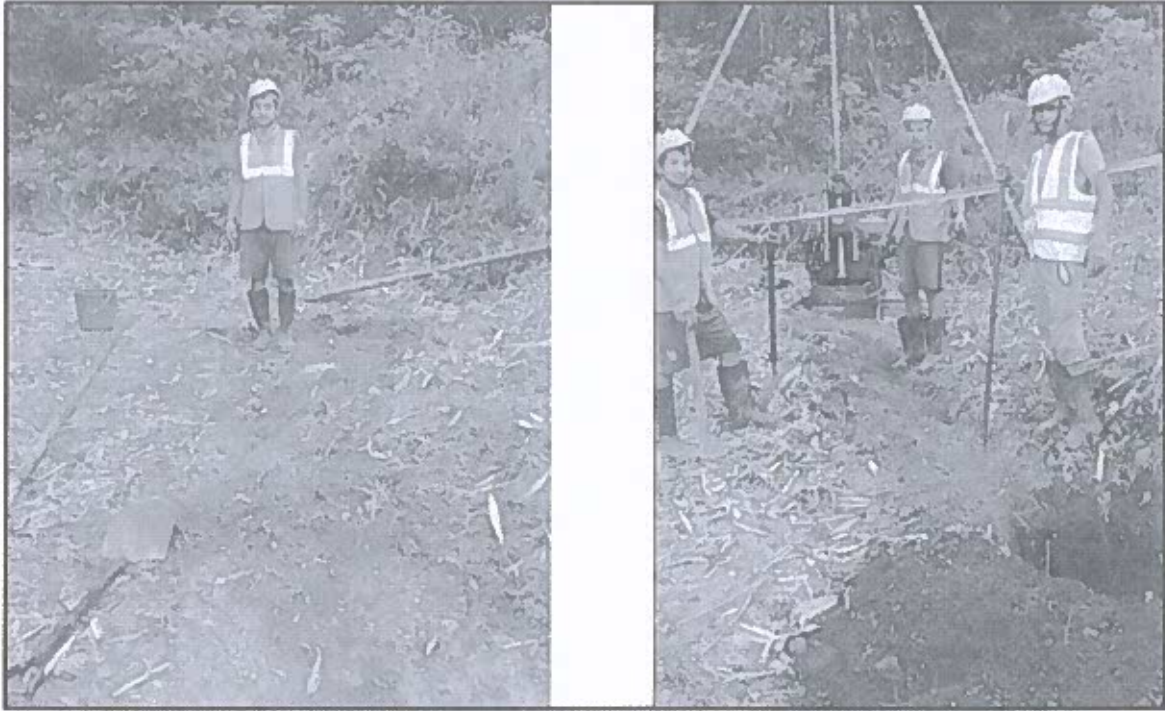
Photograph: Site conditions before Drilling at Left and Pit advancement with Completion drill hole at right at B-27
