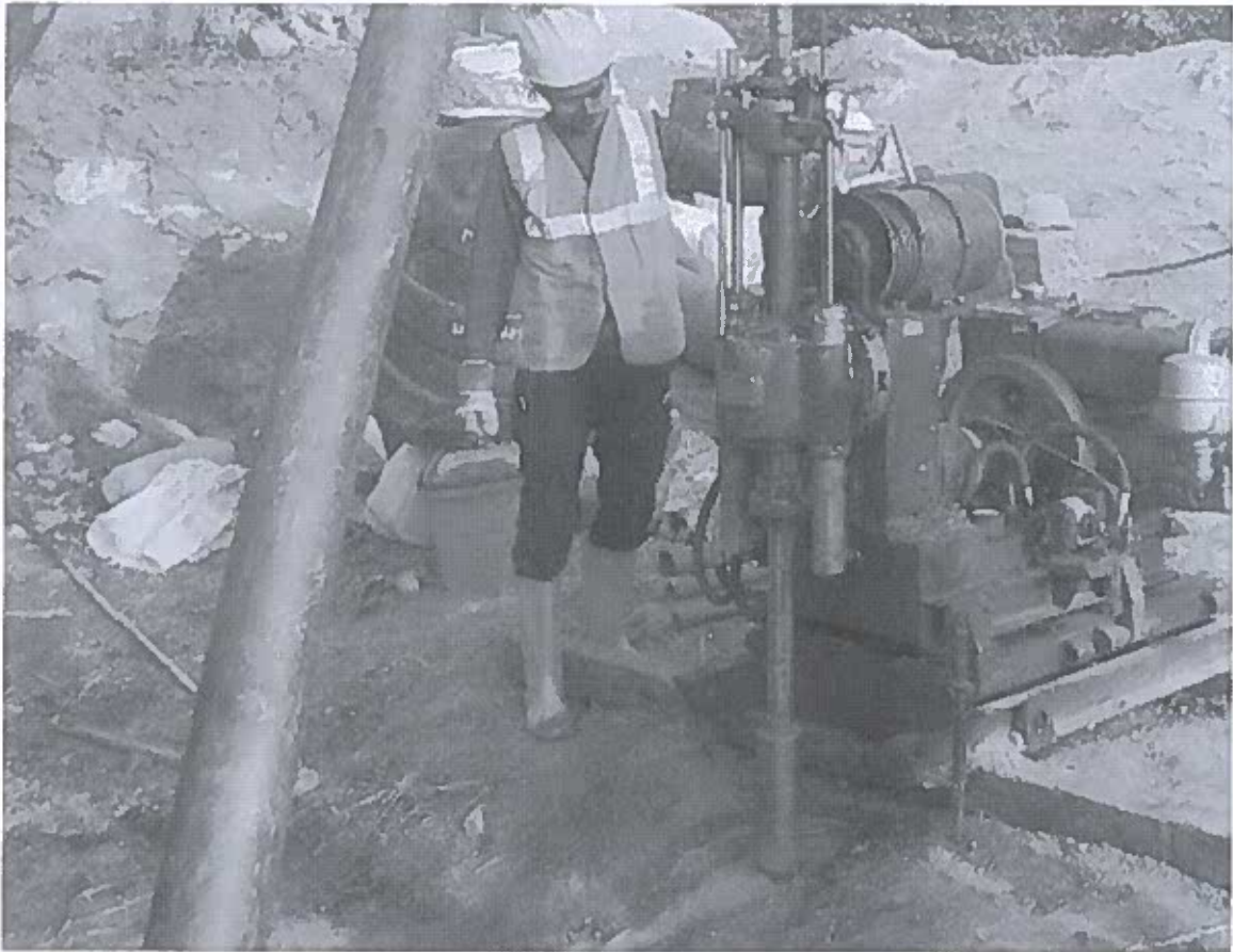
Photograph: Drilling progress work is running with greyish water return at B55
