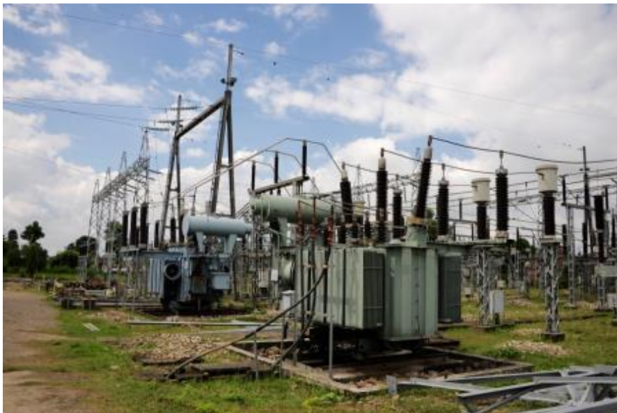
Figure 36. Existing Lamki Substation for T8 Project
